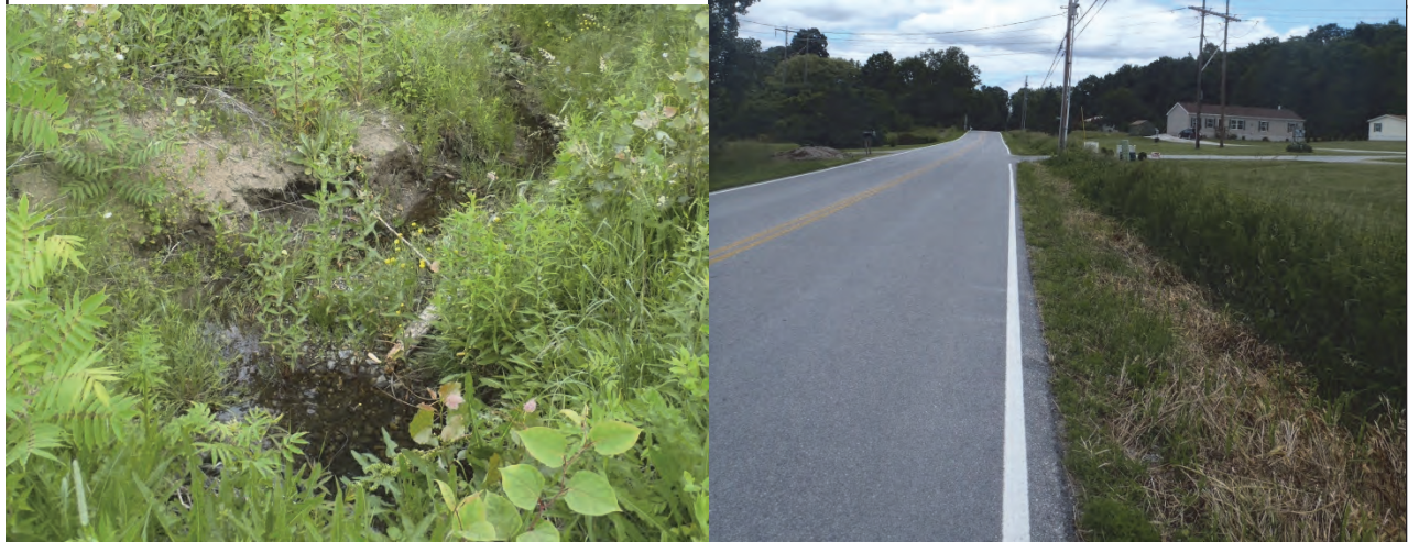
Photo 1. Active erosion at outlet to cross-culvert
