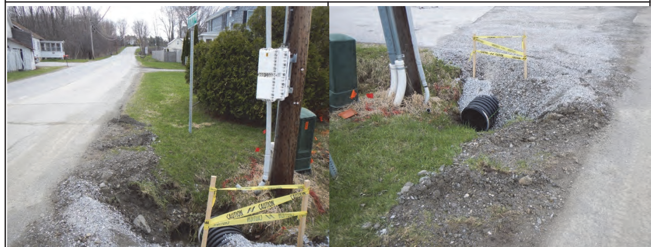
Photo 1. Culvert outlet from Church St. is buried, but visible Photo 2. Erosion will be an issue with nearby utilities
