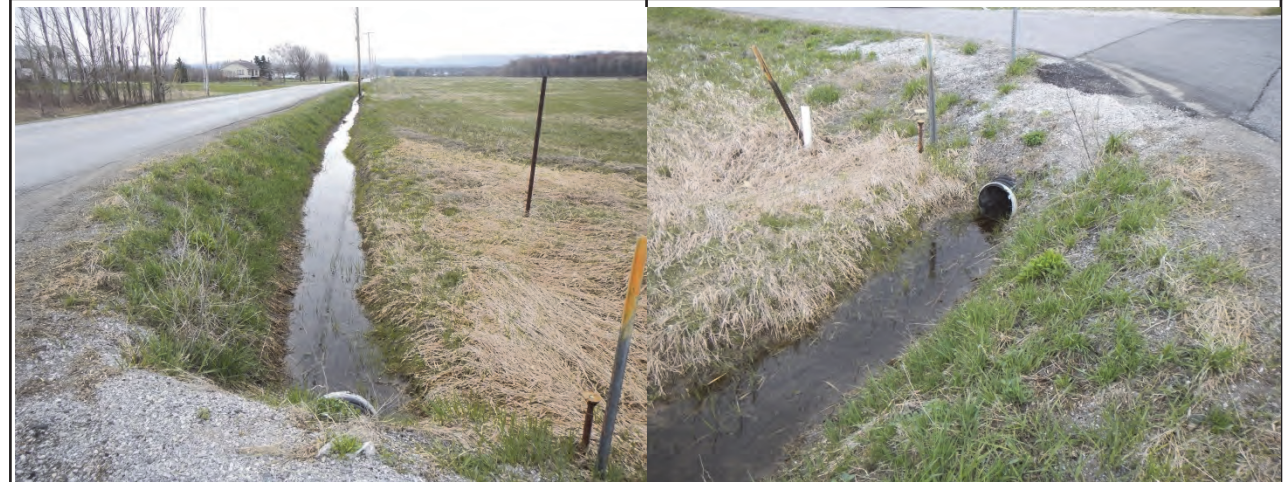
Photo 1. Narrow ditch upstream from culvert Photo 2. Culvert inlet
