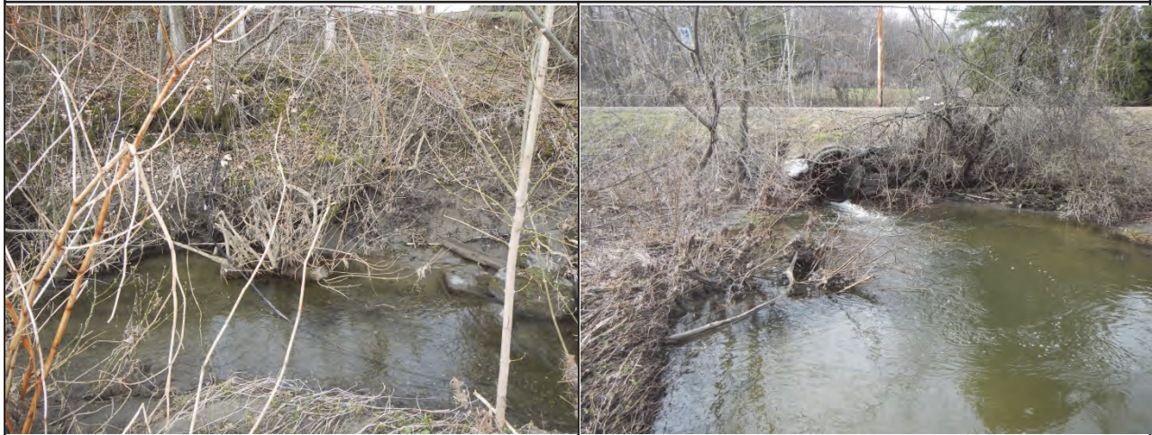
Photo 1. Bank erosion near the culvert inlet Photo 2. Large scour pool at culvert outlet.
