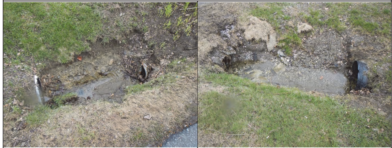
Photo 1. Discontinuous culvert sections and scour hole
