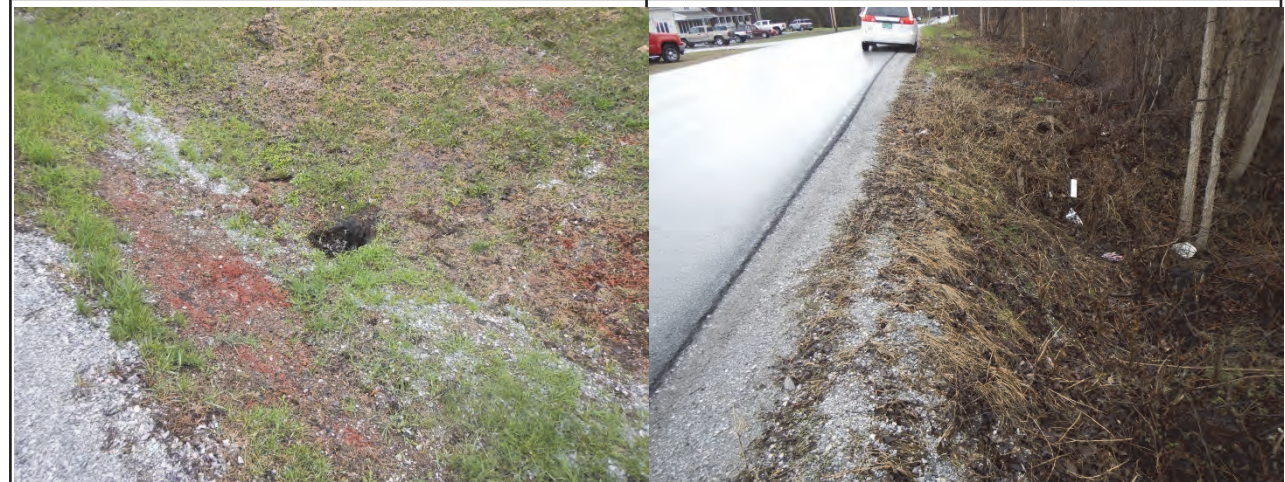
Photo 1. Culvert inlet. Photo 2. Steep bank above outlet
