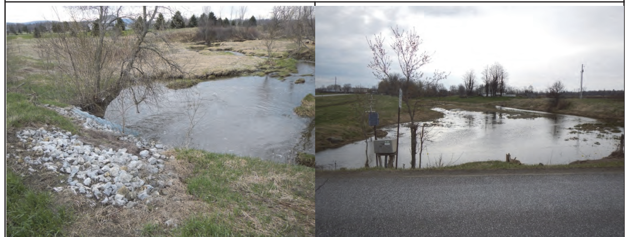
Photo 1. Scour pool at culvert outlet Photo 2. Flooded area and USGS station at inlet.
