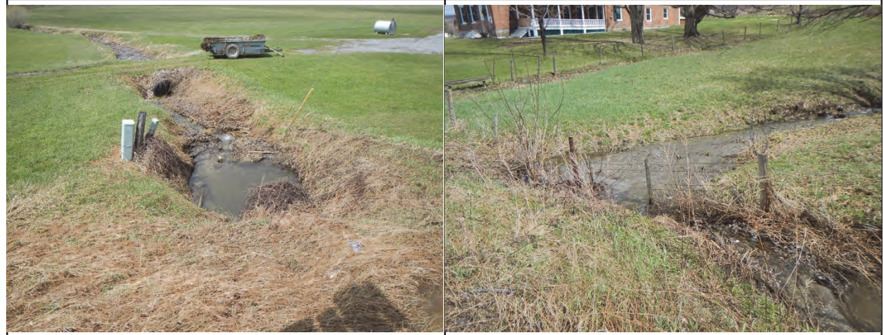
Photo 1. Scour pool at outlet Photo 2. Water ponding at inlet
