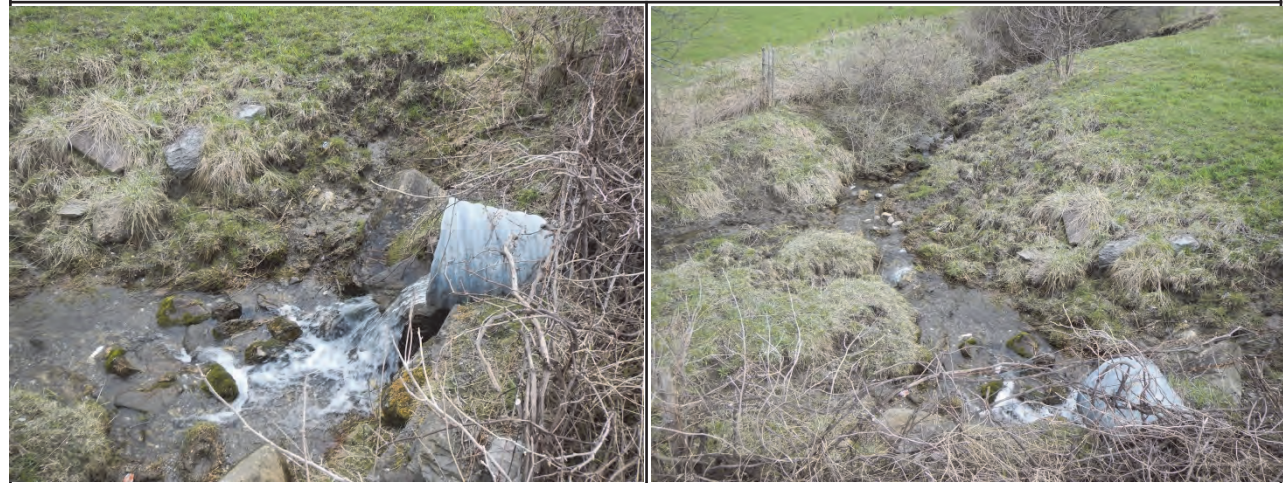
Photo 1. Culvert outlet from Church St. is buried, but visible Photo 2. Erosion will be an issue with nearby utilities
