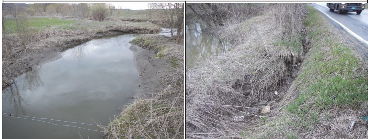
Photo 1. Scour pool at outlet Photo 2. Ditch erosion along Lower Newton Rd.
