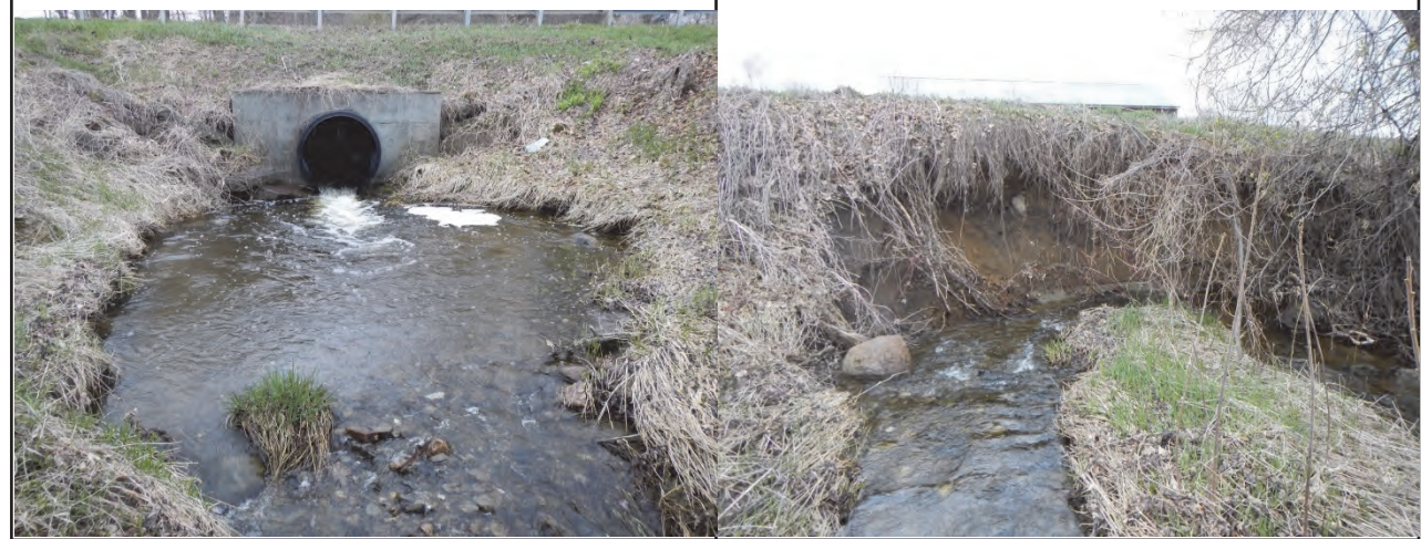
Photo 1. Scour pool at outlet Photo 2. Bank slough
