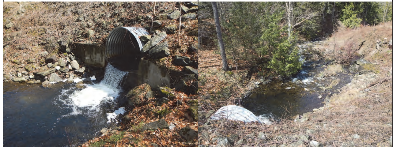
Photo 1. Perched culvert outlet Photo 2. Bank erosion downstream from culvert
