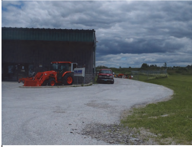
Photo 1. Downspout at Champlain Valley Equipment discharging directly onto parking lot
