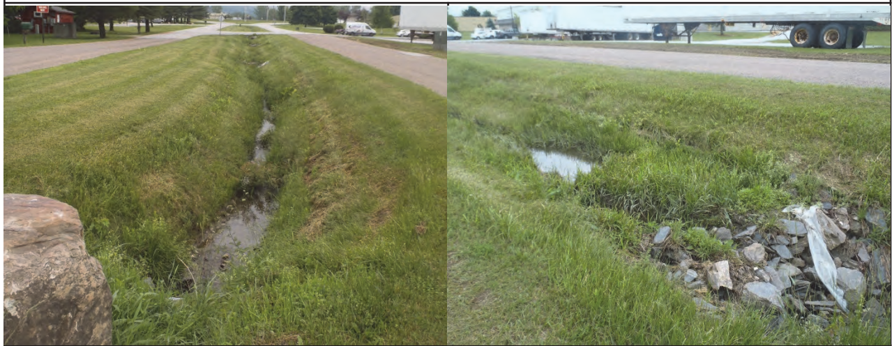
Photo 1. Swale, with some evidence of erosion
